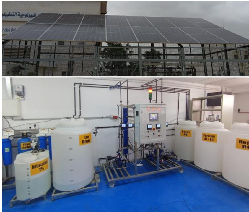
Figure 2.3.4.1 Desalination pilot and PV Solar panels at ISSBAT Facilities.
